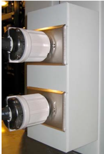
Figure 9. Facility-supplied Power Receptacles
